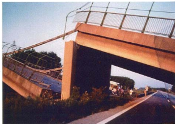
Collapse of Arifiye Overpass (Courtesy of H. Hoashi)
