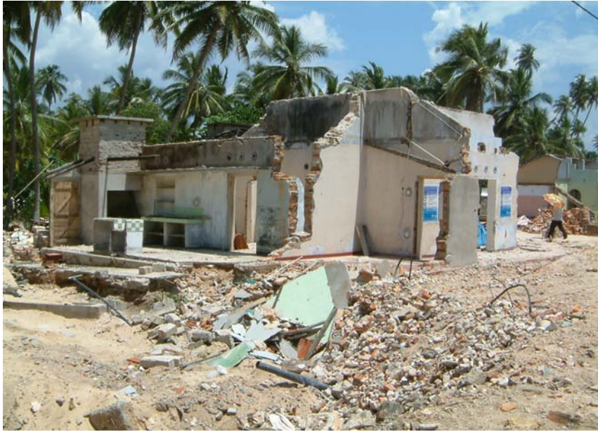
Fig. 6-3-2-6 Damaged house near the coast (Hikkaduwa)
