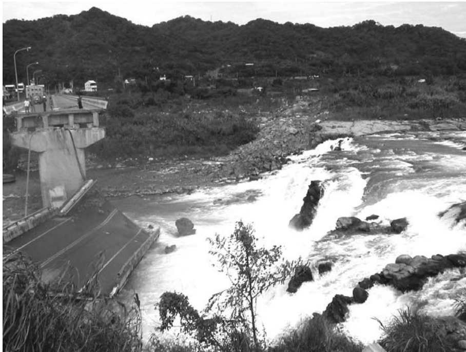
Photo 2. A destroyed bridge structure by an earthquake 1999 in Taiwan. How much was lost ? and How much do we need to for mapping of active fault distribution.? (Photo by Prof. Y. Suzuki of Aichi Prefectural University)
