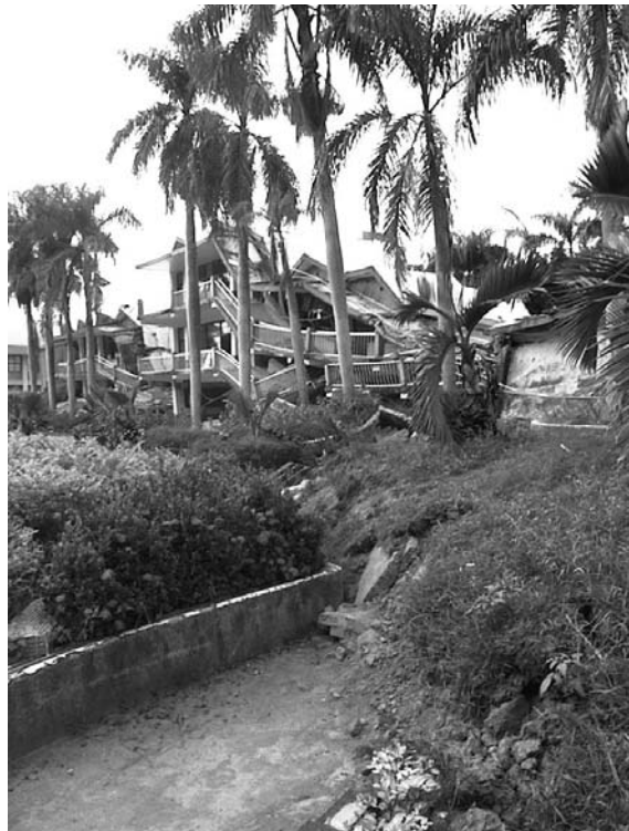
Photo 1. A destroyed school building by an earthquake 1999 in Taiwan. Fortunately earthquake occurred in a night and no children were killed in the building. (Photo by Prof. Y. Suzuki of Aichi Prefectural University)
