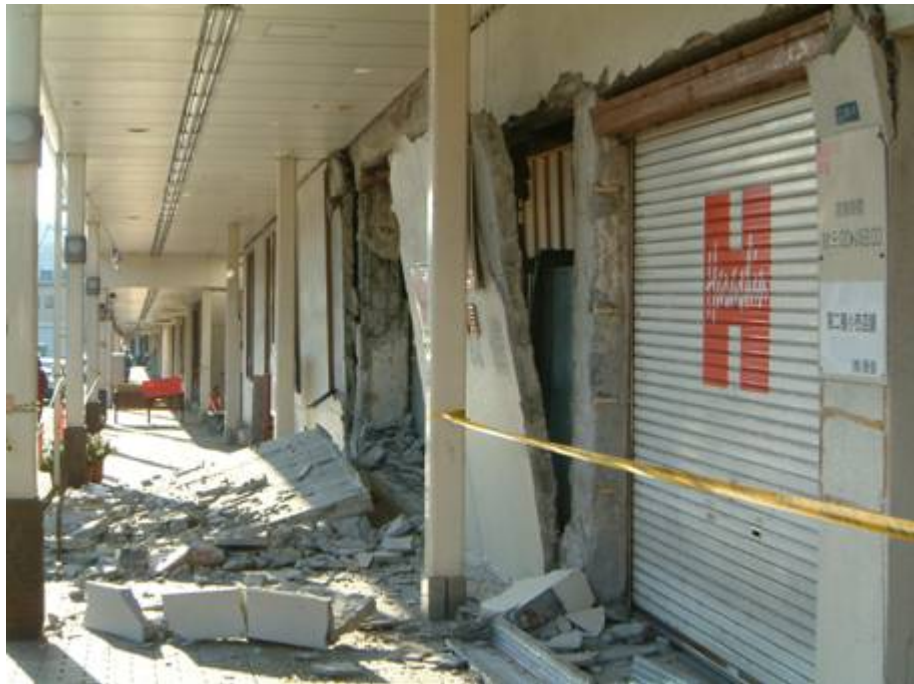
Heavily damaged store (RC structure), Ojiya city
