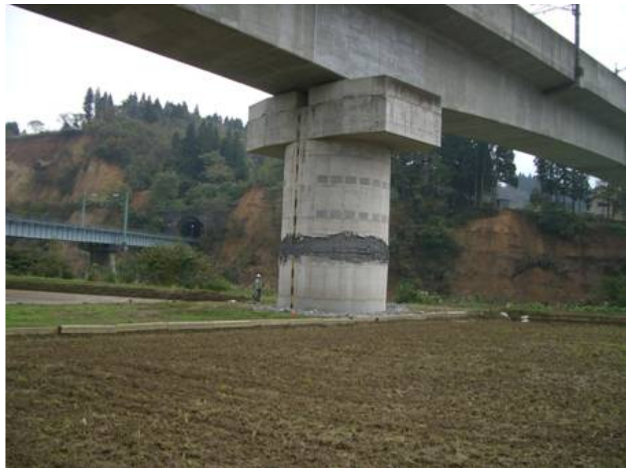
Bending fracture of bullet-train's bridge, Kawaguchi town
