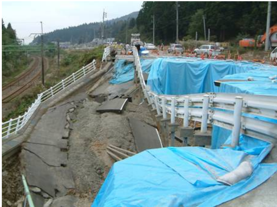
Road damage by landslide, Ojiya city
