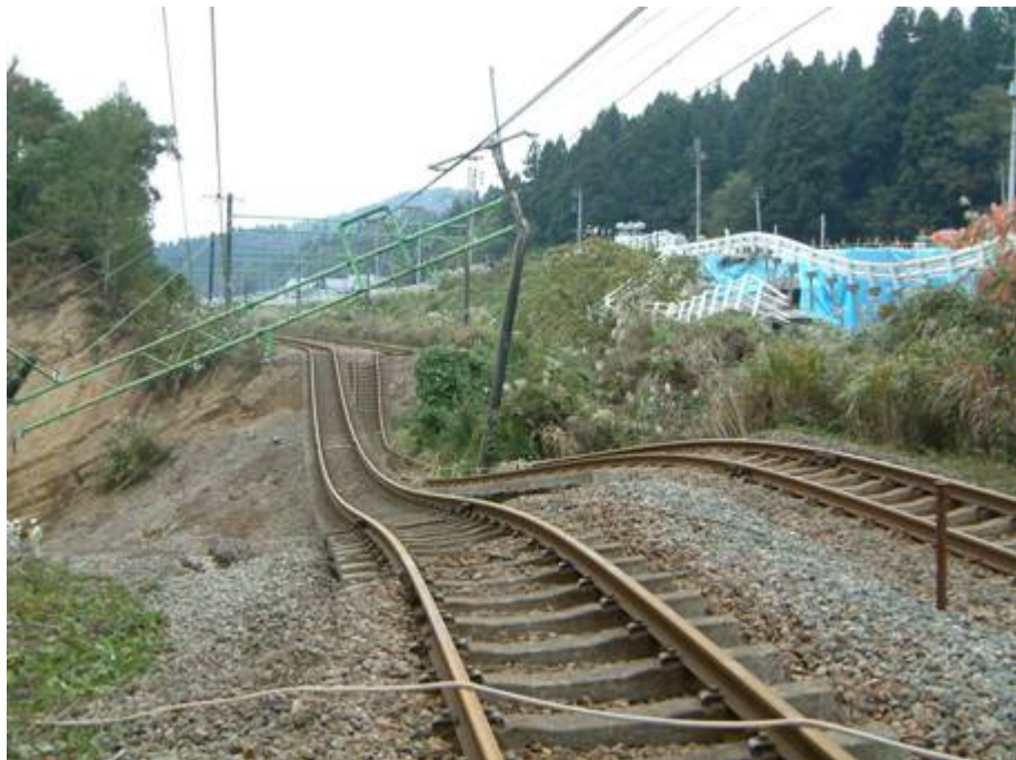
Damage to railroad by landslide, Ojiya city
