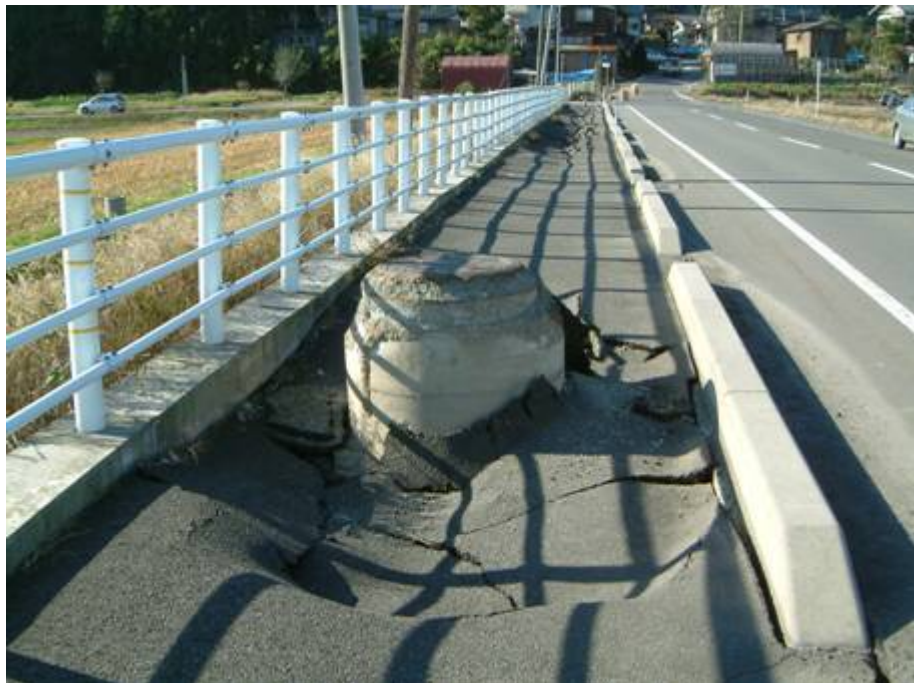
Life up of manhole by liquefaction, Ojiya city
