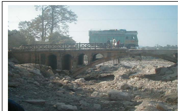
Damaged Bridge in the Khahare Khola, Mugling Narayanghat Road section.
