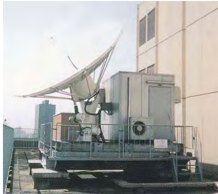
Figure shows Satellite communication facilities
