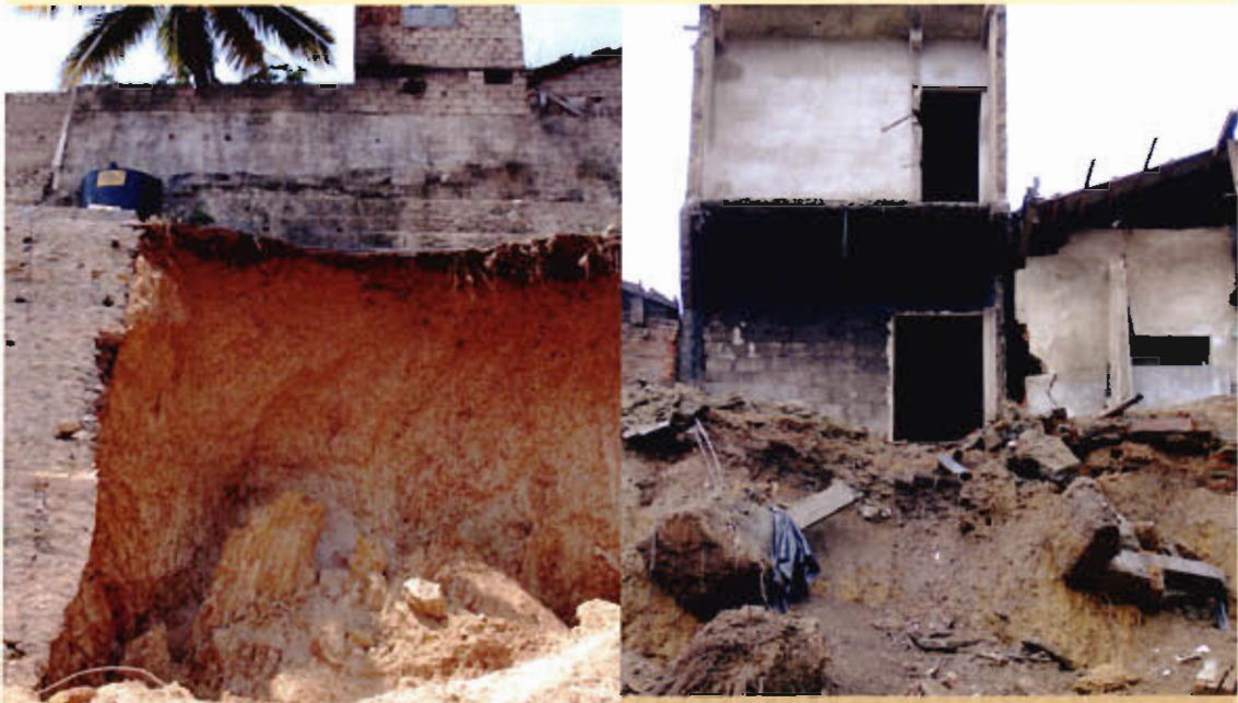
Man made cutting failure at Beruwala
